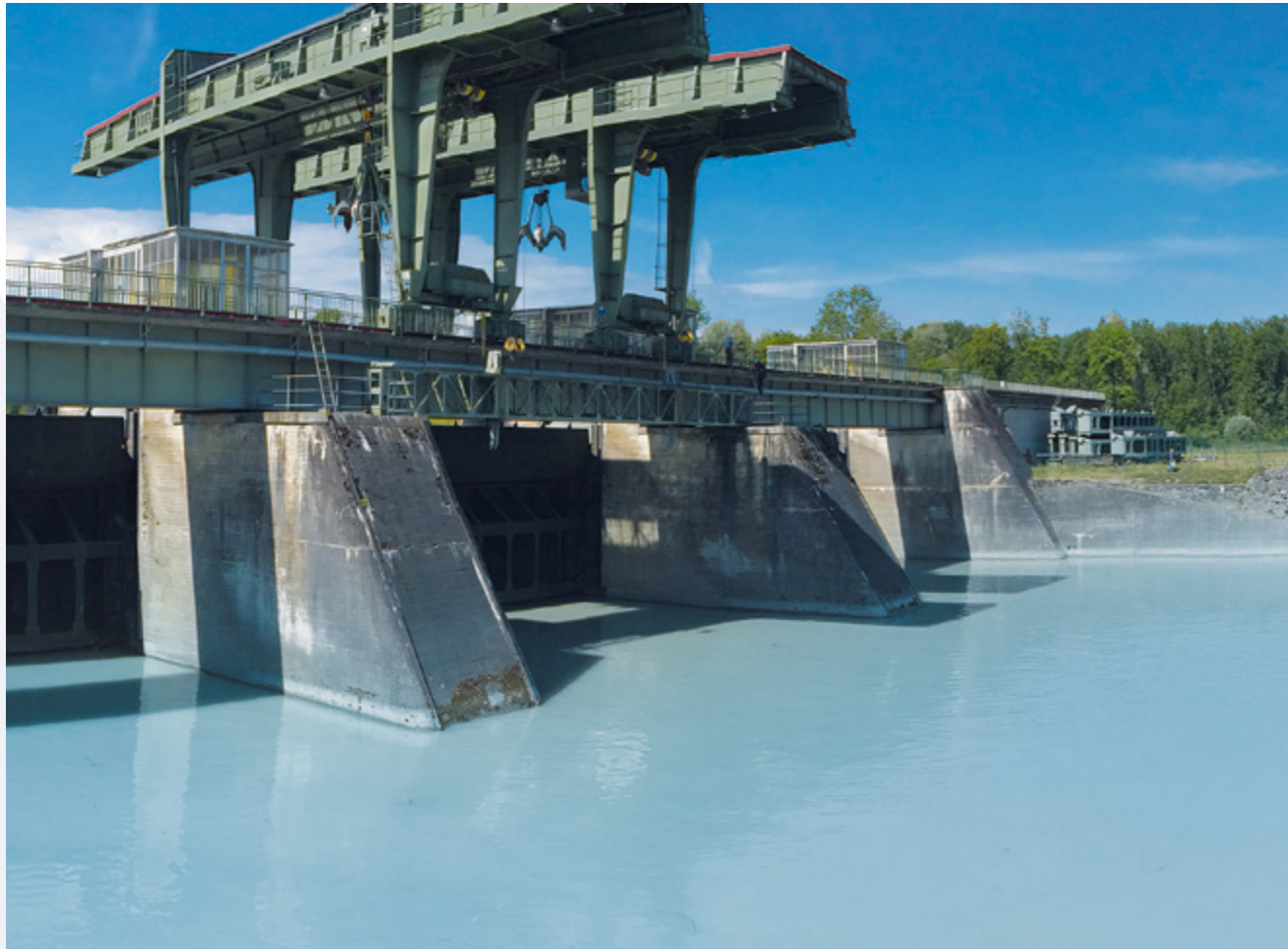
ANDRITZ Hydro will provide the instrumentation and control equipment at five hydropower stations on the Inn River.
