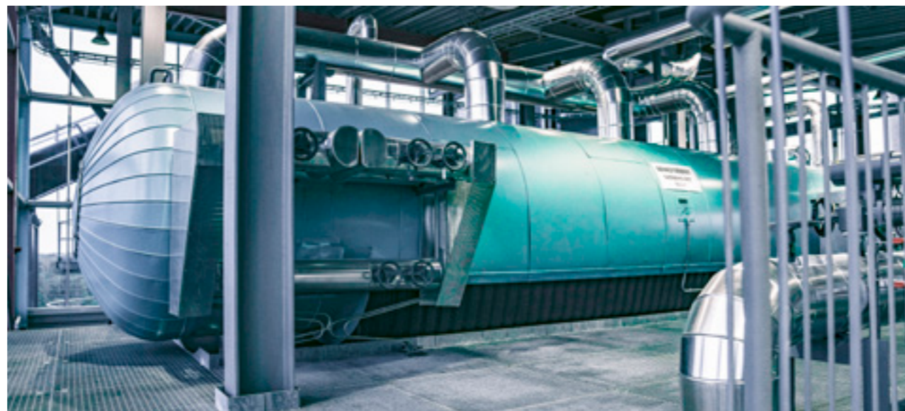
The steam temperature is around 500 °C with a steam pressure of 65 bar (a).
