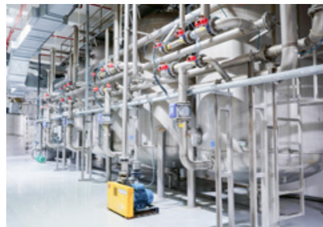
Performing filtration system designed by ANDRITZ
