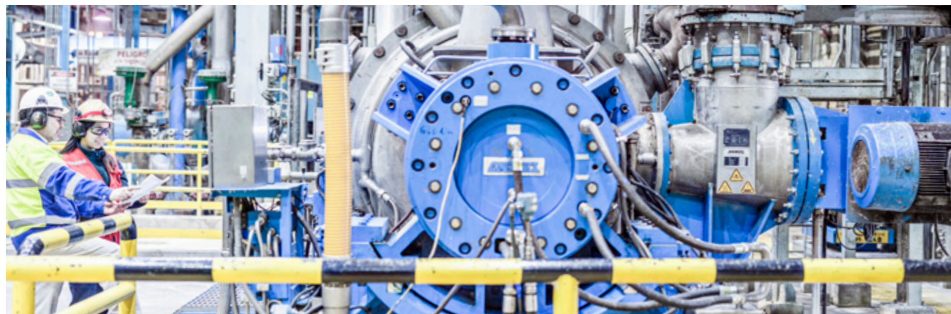
High-speed ANDRITZ HC refiner S3068 with side entry plug feeder
