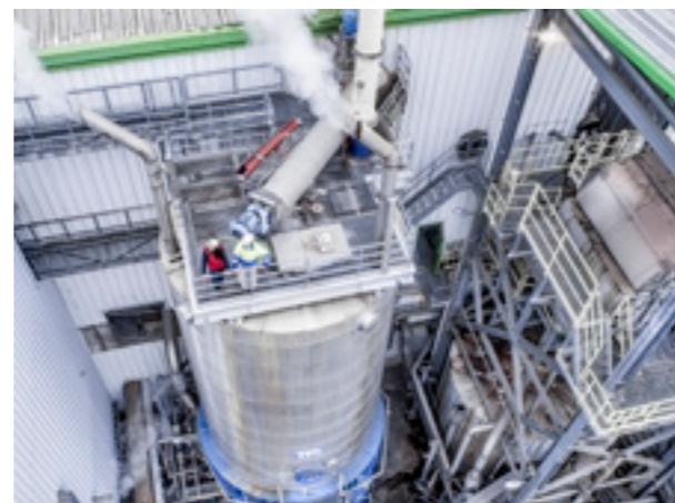
ANDRITZ PHC bleach tower with MC discharge
