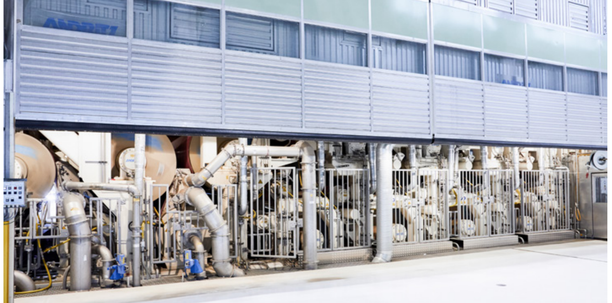
Pre- and after drying section features steel cylinders for efficient heat transfer and web stabilizers for a stable paper run.
