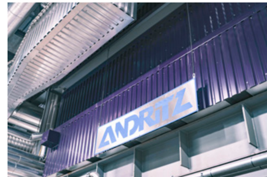
Helsingør Kraftvarmeværk specified colors of various equipment for the visual identification of different boiler parts.
