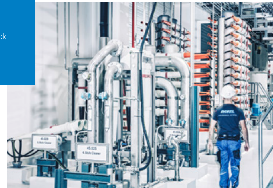
Five-stage cleaner system for the new PM3
