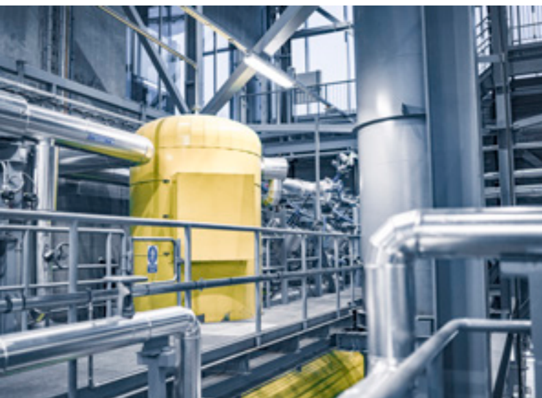
The boiler burns wood-based biomass, which consists of forest residues, bark, sawdust, and woodchips.
