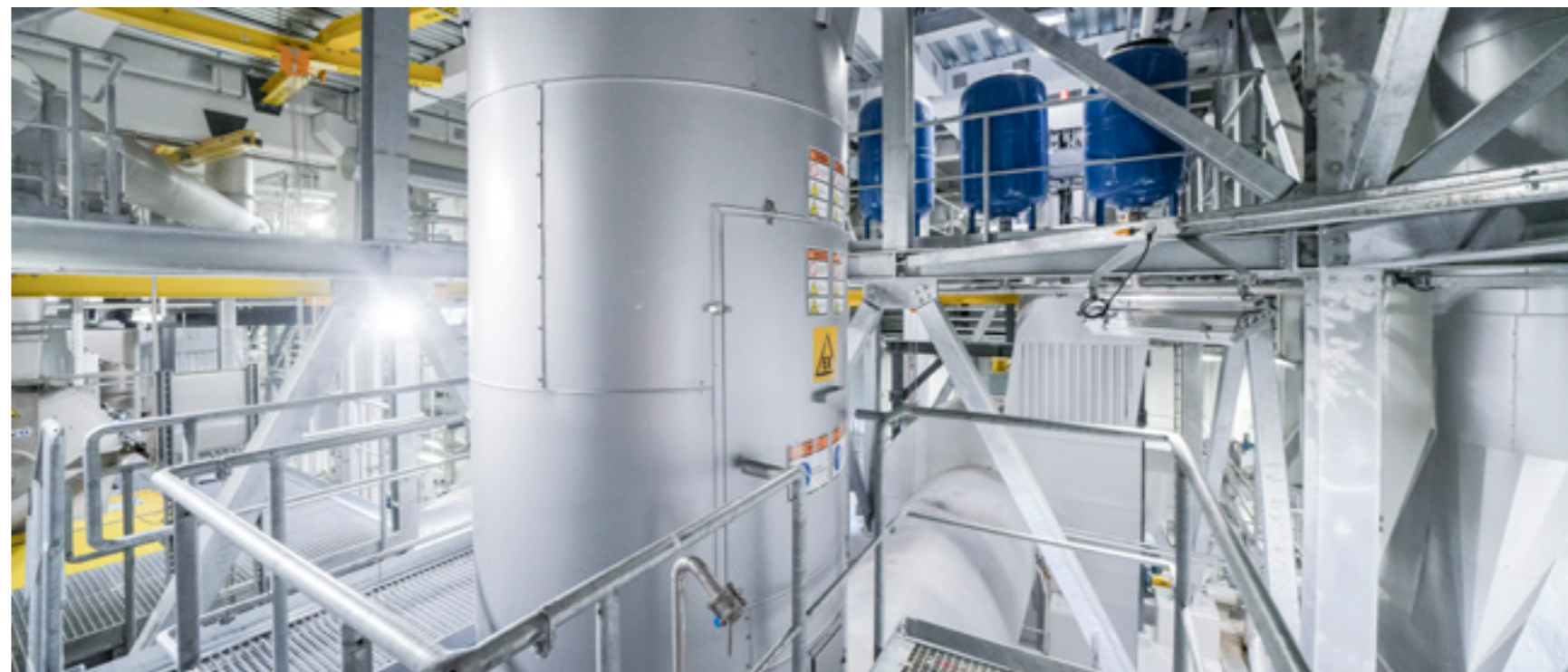
Equipment is easily accessible for service and maintenance, despite the tight space available.
