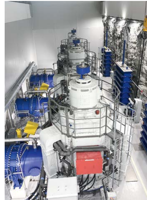
Powerhouse of Tolga. The new run-of-river power plant is equipped with three identical 15 MW compact Francis turbines.
