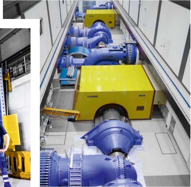
With four generating units, Wehr is the biggest power plant in the portfolio of Schluchseewerk AG and provides crucial grid balancing services.
