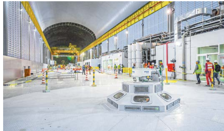
The main powerhouse is over 270 m long and features six units, each with a rated power of 335 MW.
