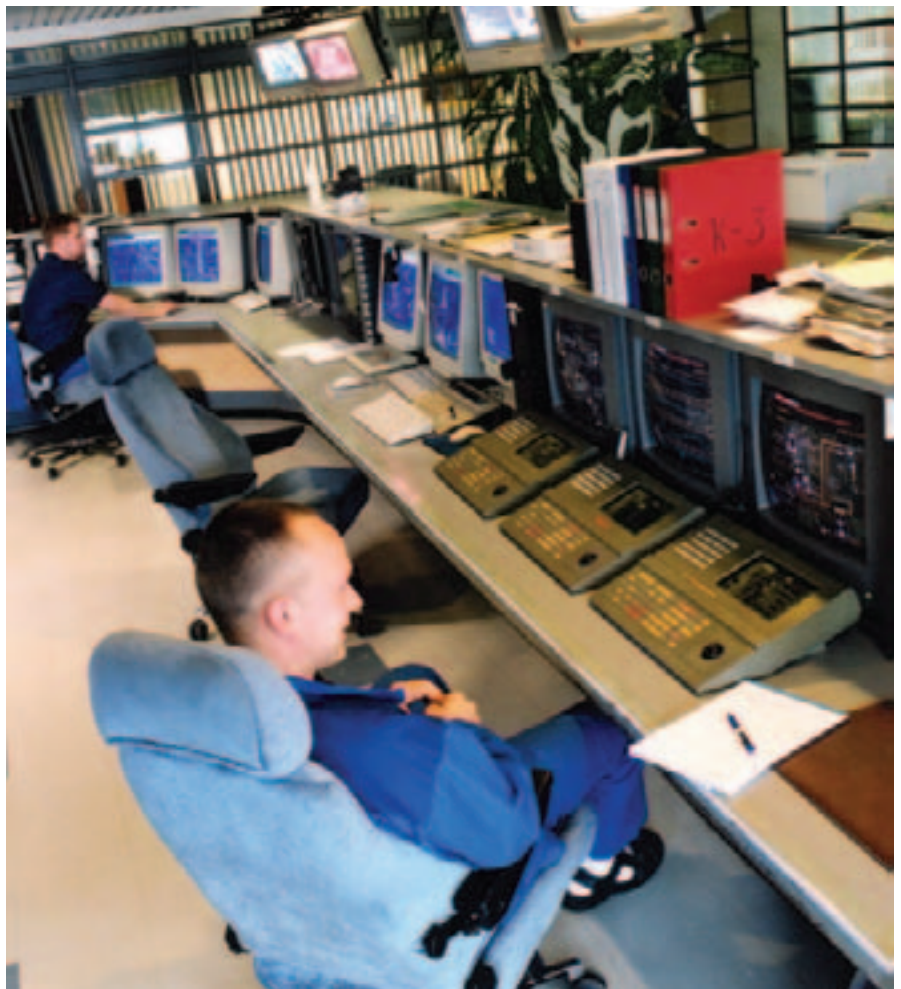
The modern fiberline control room for wood processing, hardwood pulp and softwood pulp lines at Kuusankoski. Esa Vanhalakka is the operator in the foreground, and Niko Saarinen is in the background.
